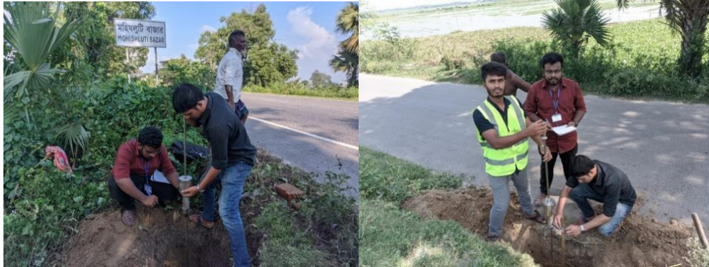
Fig. 4: Dynamic Cone Penetration test on the Hatikumrul-Bonpara highway (N507) (Coordinates: 24°22'26.3" N 89°23'02.8" E).
